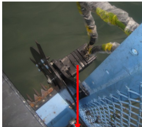
Cutting wheel driving motor
