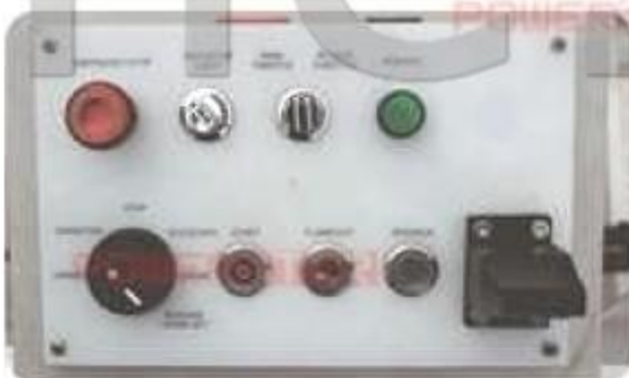
PLC control box in cage
