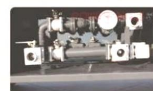
valve system with flow meter
